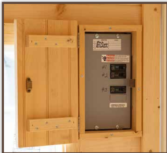
Breaker Box with Breakers
