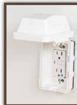
Exterior GFCI Receptacle with In Use Cover
